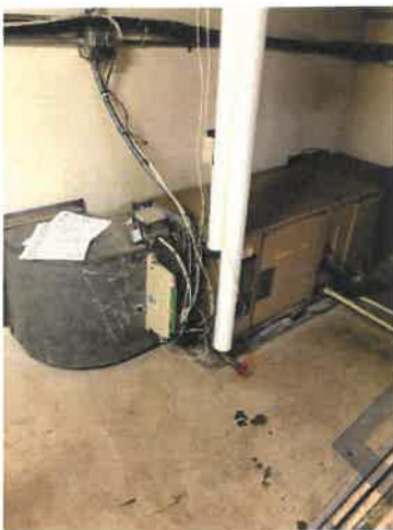
Small Air Handler
