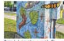
Painted electrical box example (E)
